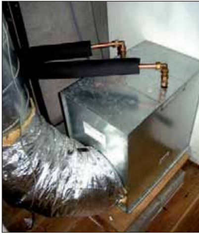
Water to air heat exchanger unit. Source: MosArt Architecture
