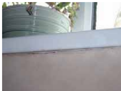
Smoke test illustrating air leakages below a window sill Source: MosArt Architecture
