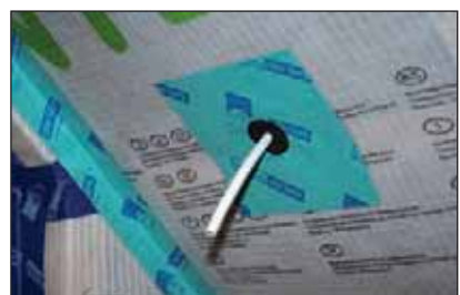
Use of rubber gasket to seal a penetration of the airtight membrane. Source: MosArt Architecture
