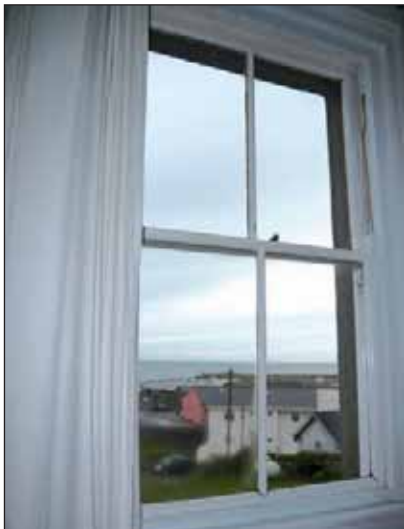
Traditional sash window with mullions and stanchions which reduce solar gains and create a thermal bridge from outside to inside
