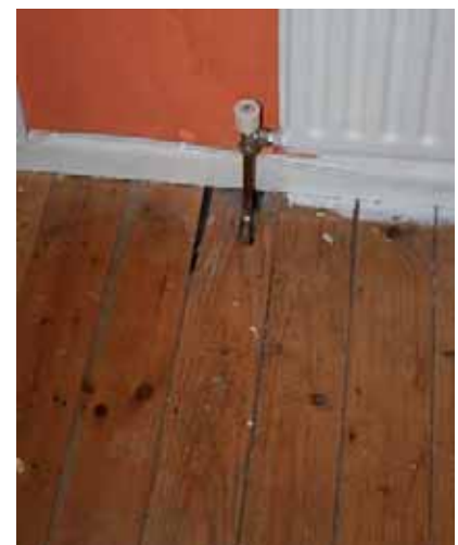
Leaky floor construction Source: MosArt Architecture
