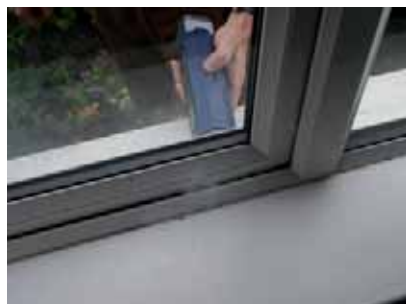
Smoke test clearly highlights poorly sealed windows Source: MosArt Architecture
