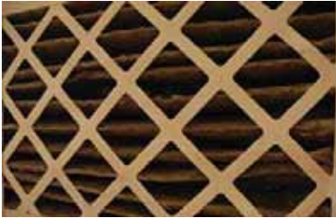
Dust laden used air filter. Source: MosArt Architecture.
