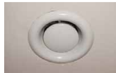
Ceiling air supply vent. Source: MosArt Architecture.
