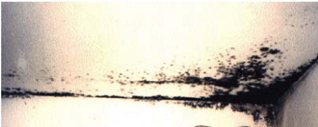
Figure 91 - Mould at external wall and ceiling junction
