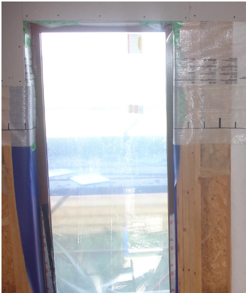
Figure 12 Sealing under way at junction of timber frame wall and external wall ope
